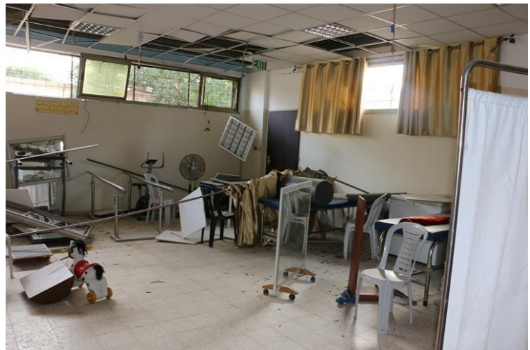
Palestine Avenir for Childhood Foundation (PACF) – Cerebral Palsy Center exposed to severe damages due to an Israeli airstrike nearby the building. Photo credit: PACF
